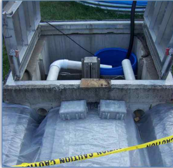
Figure 7. Parking lot drain outlet into sampling box for rainwater collection.
